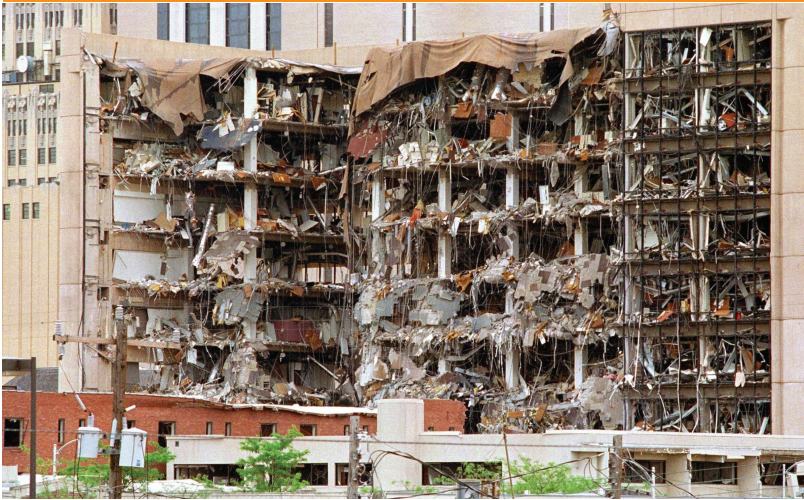
Murrah Federal Building, Oklahoma City, after the bombing on 19 April 1995.
